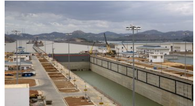
Expanded canal opens Asia market to U.S. shale gas Canal route shortens trip by one-third
